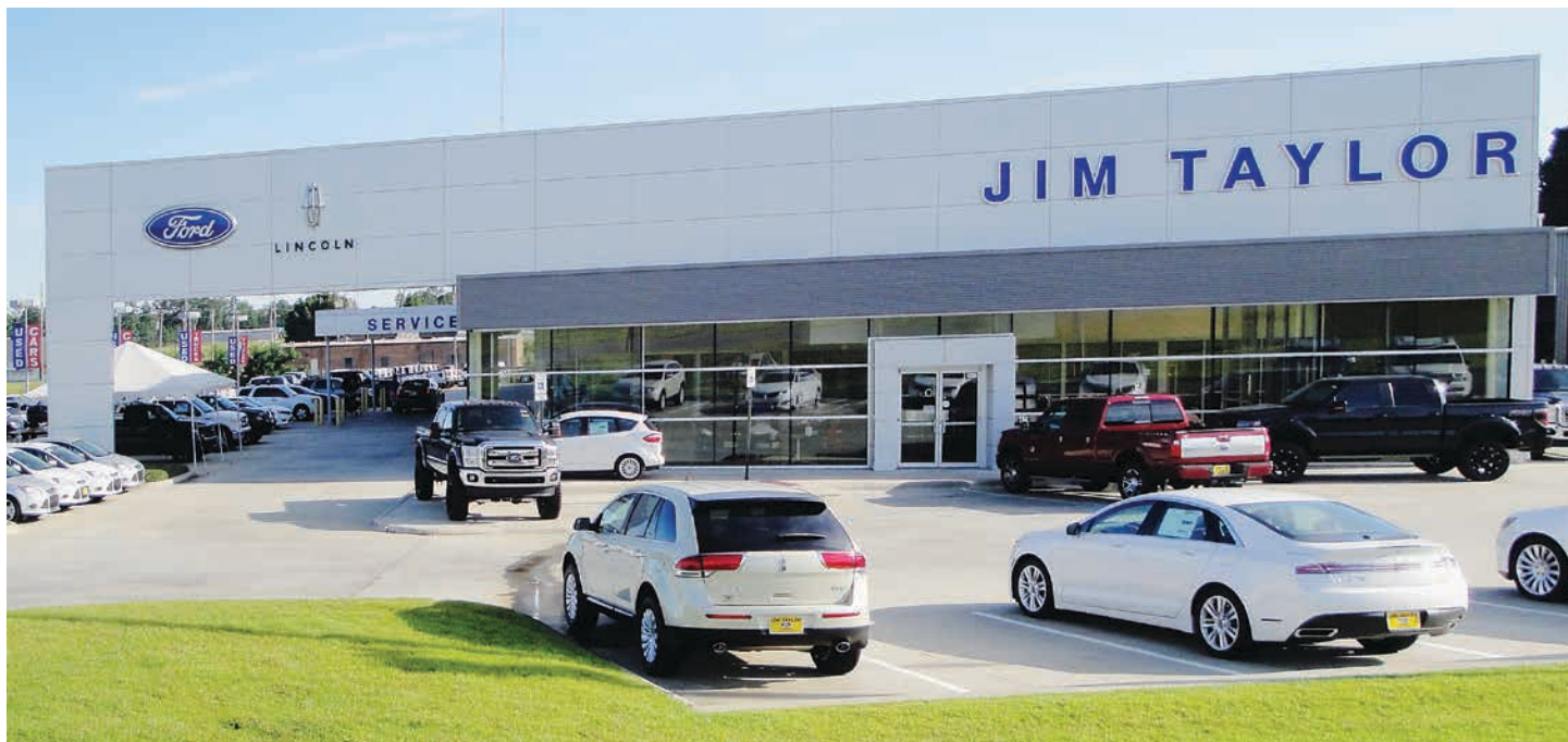
New auto dealership and shop addition constructed for this valuable client in a highly visible location along I-20 in Ruston.
